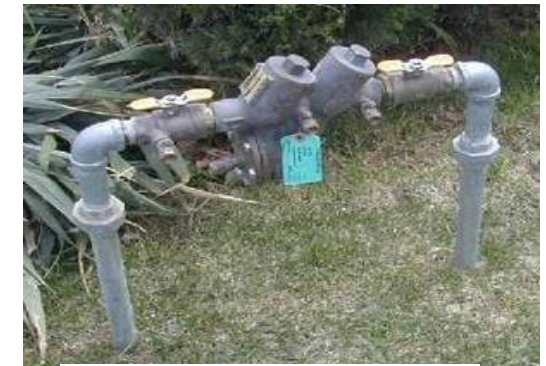
Common residential backflow preventer
